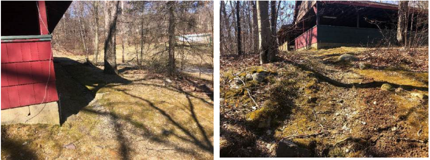
Photos 104-105. Erosion along the outside of the pavilion from the roof runoff
