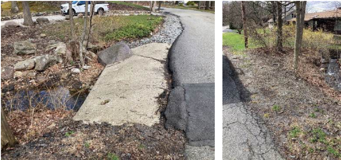
Photos 51-52. Stream crossing on the west side of Kitchell Lake Drive East
