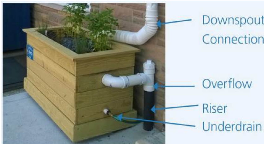
Photo 136. Downspout planter, Source: Phillywatersheds.org
