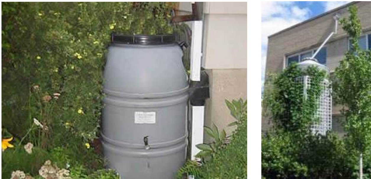
Photo 134-135. Rain barrel (left) and cistern (right), Sources: CTDEEP (left) and USEPA (right)
