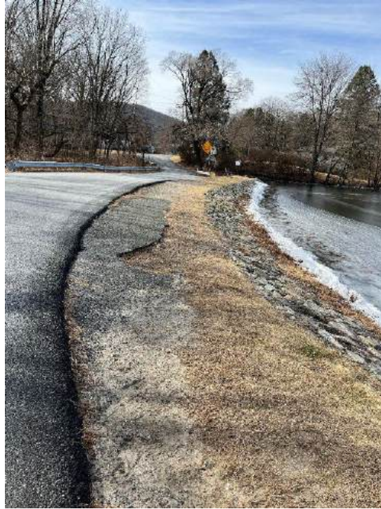
Photo 124. Evidence of sediment from the road and existing compacted grass and stone shoreline
